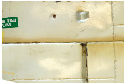
Corroded plate underside
